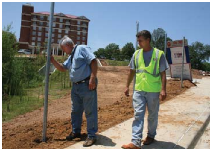
Morris Horn, University of Mississippi (left) and Freddie Gurley, UtiliQuest, check the progress on the 7000’ security fence on the Ole Miss campus.
